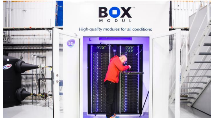
Edge, wind tunnels and liquid cooling test beds
